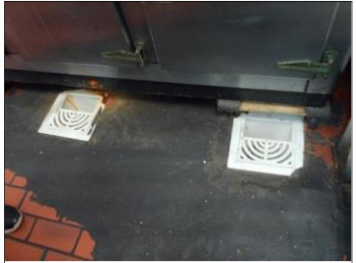
74. Kitchen area floor drains; Note flooring sealing repairs
