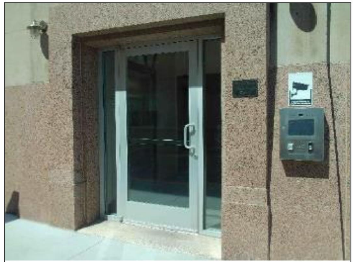
10. Northeast common building entrance leading to the kitchen access door and basement stairs
