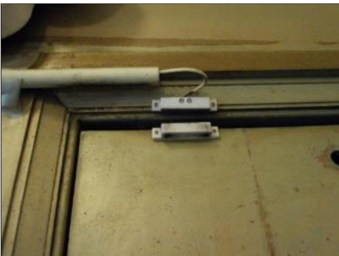
77. Typical security system door sensor
