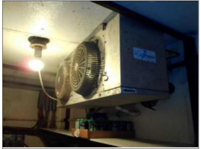
20. Beer cooler refrigeration unit to remain in the basement
