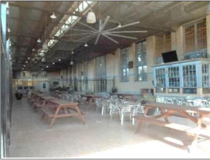
37. Overview of the south exterior patio area; Note current tenant-owned tables and chairs to be removed by the outgoing tenant
