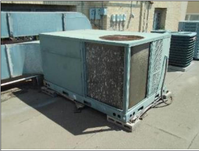
61. Goodman 2008 vintage 5-ton RTU on the open patio area roof that serves the dining/bar area; Note hail damaged coils
