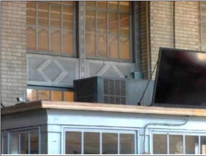
43. 2.5-ton packaged HVAC unit serving the service/bar kiosk and interior dining/bar area to remain
