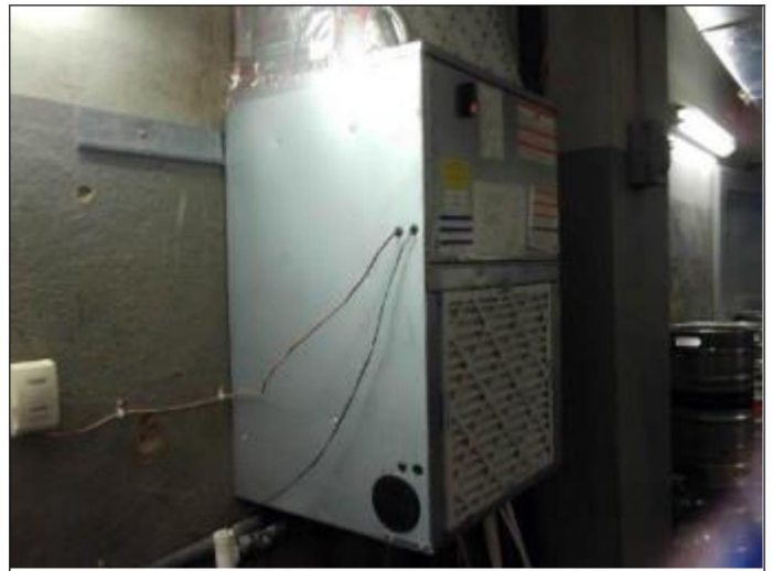
34. Split system HVAC condensing unit in the basement (HOA owned)
