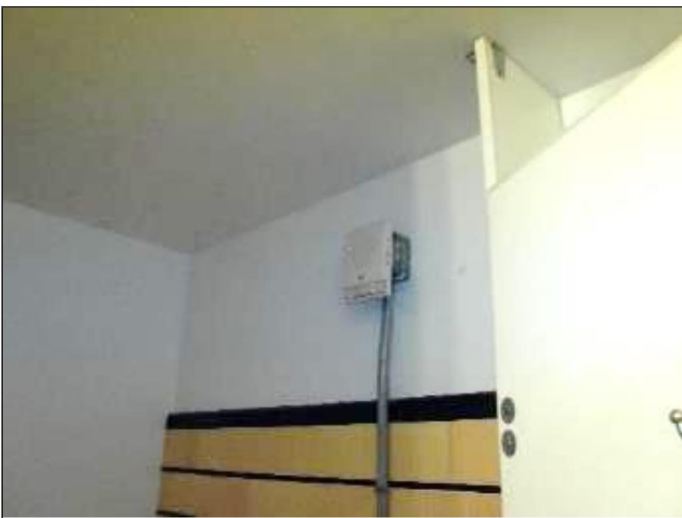
83. Only the women's restroom was provided with a fire alarm system audible/strobe unit
