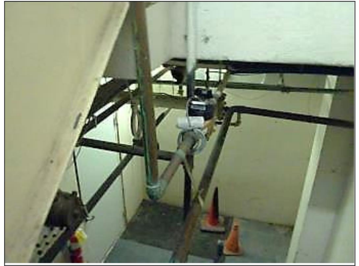
14. Main domestic water supply line and meter in the basement
