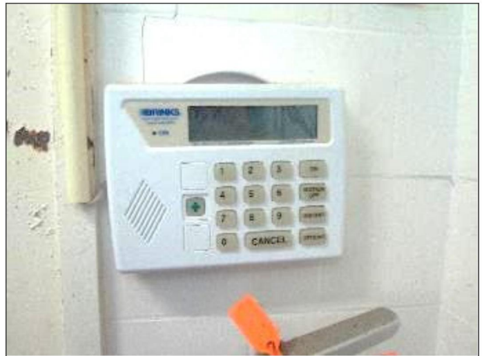
76. Security system control pad
