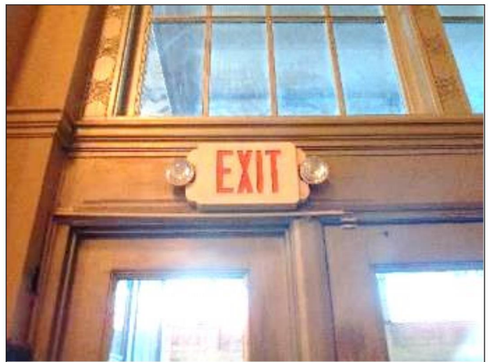
84. Lighted exit sign with emergency lighting
