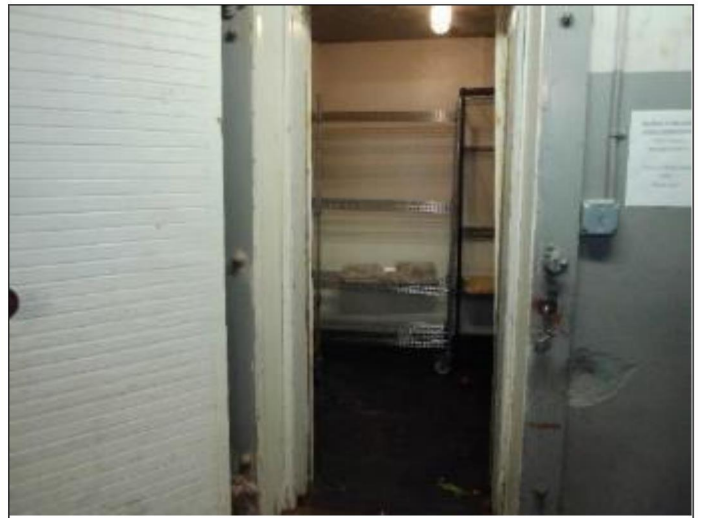
22. Food walk-in cooler to remain in the basement
