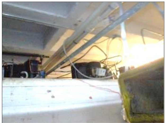
54. The refrigeration compressor unit for the bar area wine cooler is located in the basement
