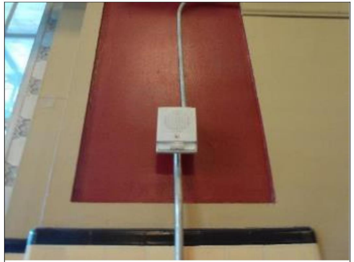
82. Typical fire alarm system audible/strobe unit
