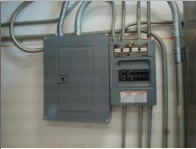
73. Kitchen area electrical panels
