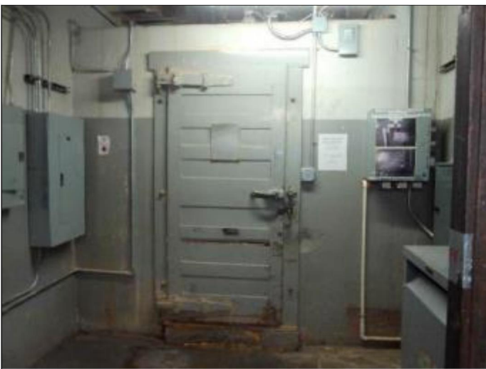
17. Beer walk-in cooler to remain in the basement
