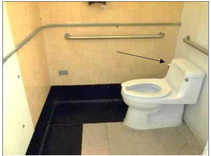
58. The Men's toilet flush valve is on the wrong side of the tank
