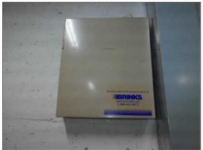
30. Subject property Brinks security system electrical control panel to remain in the basement
