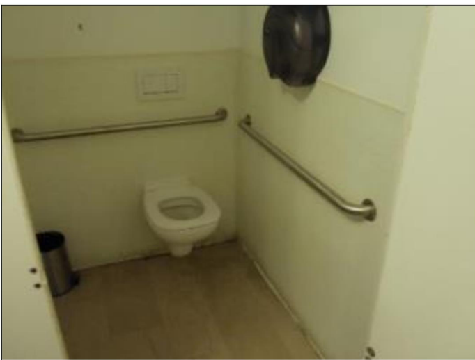
59. The toilet paper dispensers are not installed at compliant heights in both restrooms
