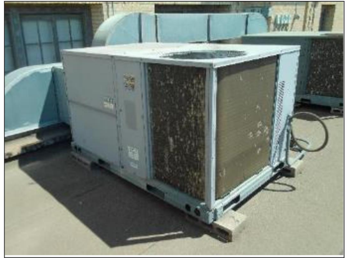
62. International. Comfort Products, LLC 2011 vintage 6-ton RTU on the open patio area roof that serves the dining/bar area; Note hail damaged coils
