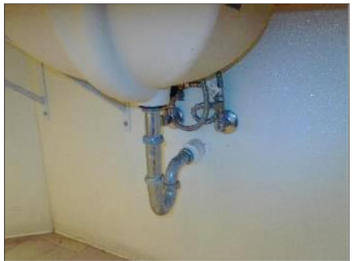
60. Both restrooms are missing compliant under sink pipe wraps
