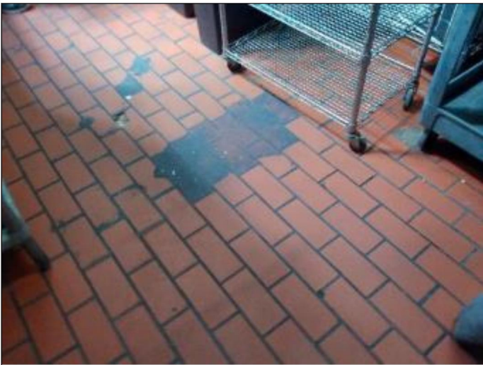
75. Typical flooring conditions in the kitchen area
