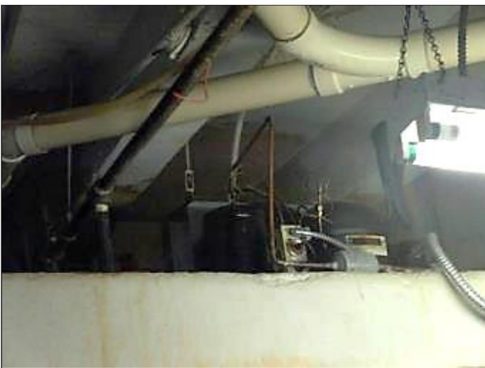
23. Food cooler 0.75-HP refrigeration compressor to remain in the basement
