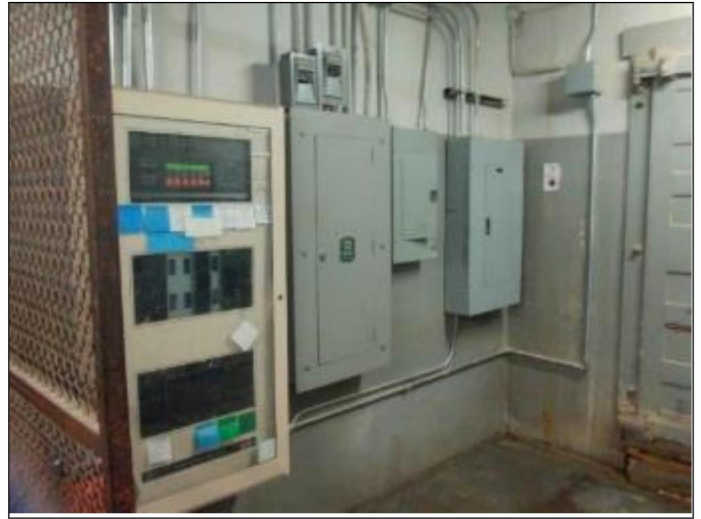
32. Main HOA owned FACP and HOA owned electrical panels in the basement
