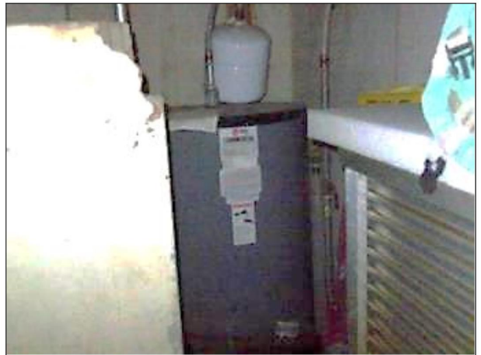
16. 120-gallon electric water heater to remain in the basement
