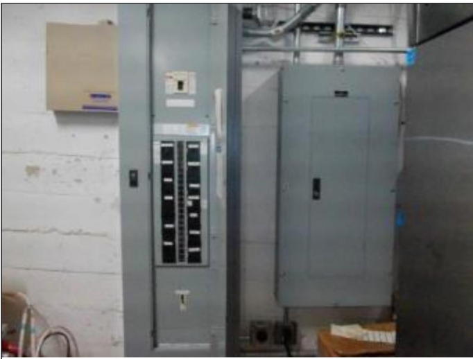
27. Subject property electrical panels in the basement
