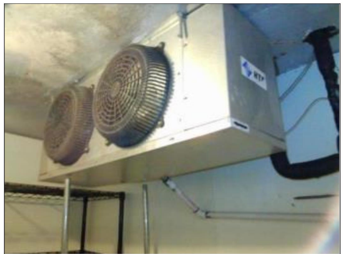
24. Food cooler refrigeration unit to remain in the basement
