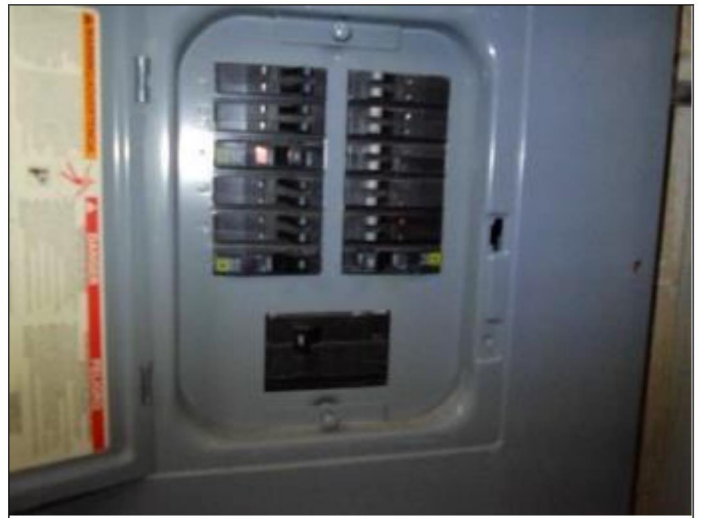
28. Subject property electrical panels in the basement
