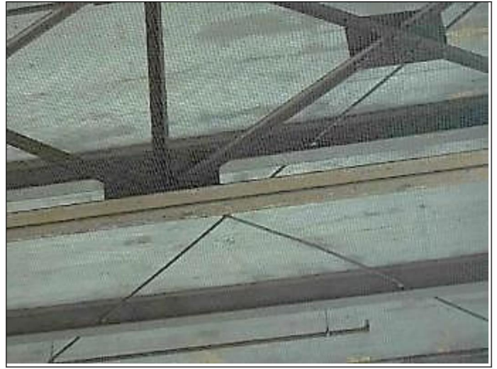
38. South exterior patio area bird netting on the exposed roof structure to remain
