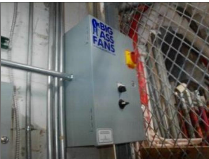
29. Subject property 'Big Ass Fan' electrical control panel to remain in the basement
