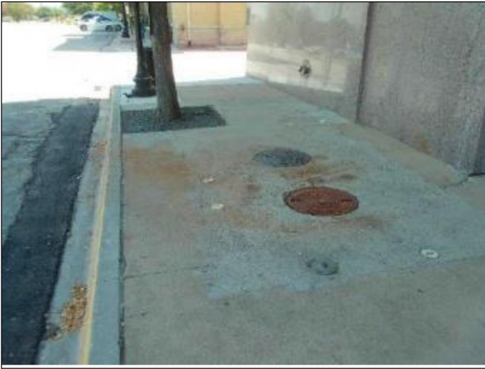
7. Location of the 1,000-gallon grease trap to remain at the northeast corner of the building
