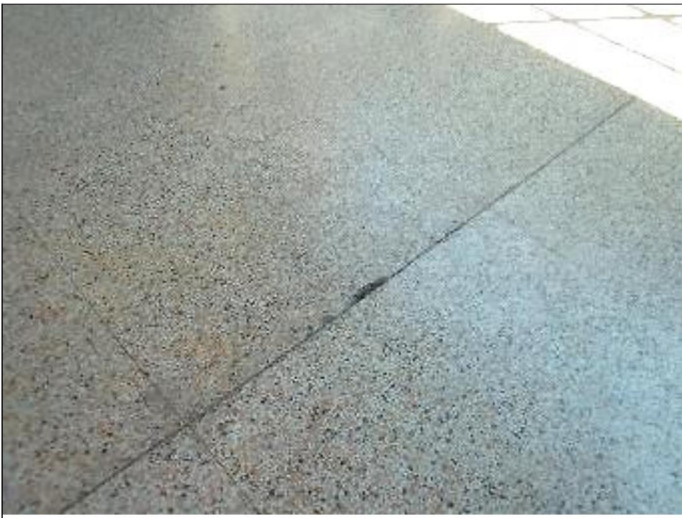
81. Isolated areas of minor damage to the exterior patio area epoxy flooring were observed
