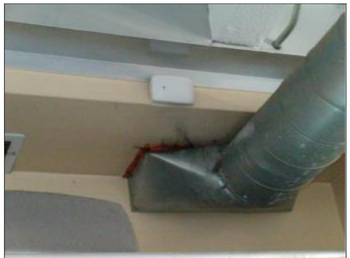
78. Typical security system kiosk sonic glass break sensor
